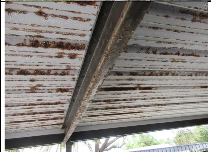
11. Observed severe rusting along Northwest and Center West Carports. (Continuous Monitoring Recommended)
