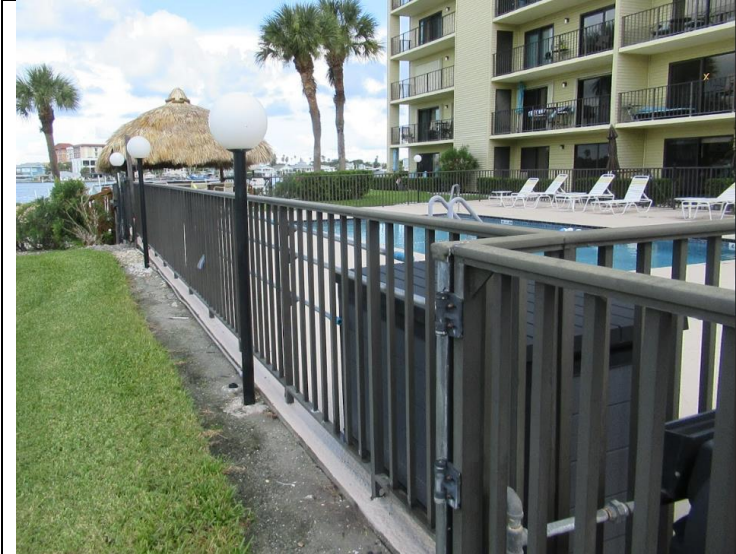
10. Common area walkway and pool railings.
